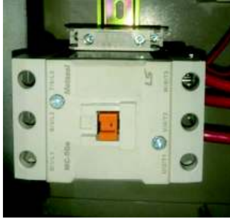
Figura 9 Contactor principal de 50 (A).
