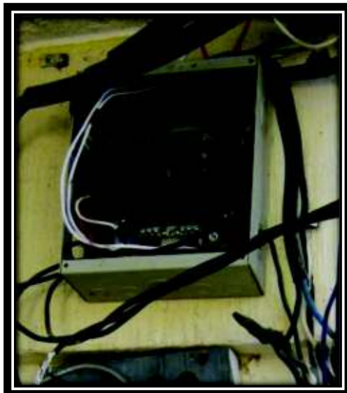
Figura 3.9 Tablero principal B.
