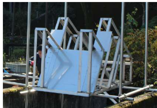
The steel plate(Block Plate) blocks the flow of water to level up the water surface to the hydraulic head.
