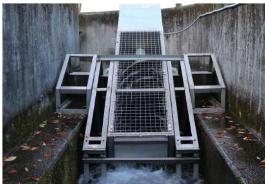
For stability Foundation Frame is supported on both sides by additional frame work to fit the structure of the channel.
