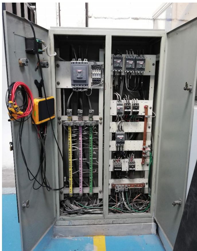
Figura 3.6. Tablero de control principal
