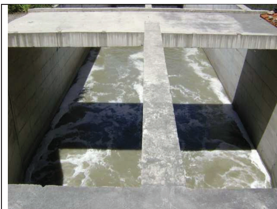
Colector El Batán (Agua Residual)
