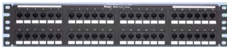
Figura 3.11 Patch Pannel de 48 puertos [6]
