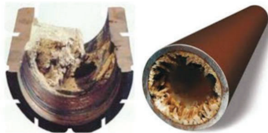
Figura 26. Tubería con incrustaciones (EMEC, The Egyptian Mud Engineering and Chemicals Company, s.f.)
