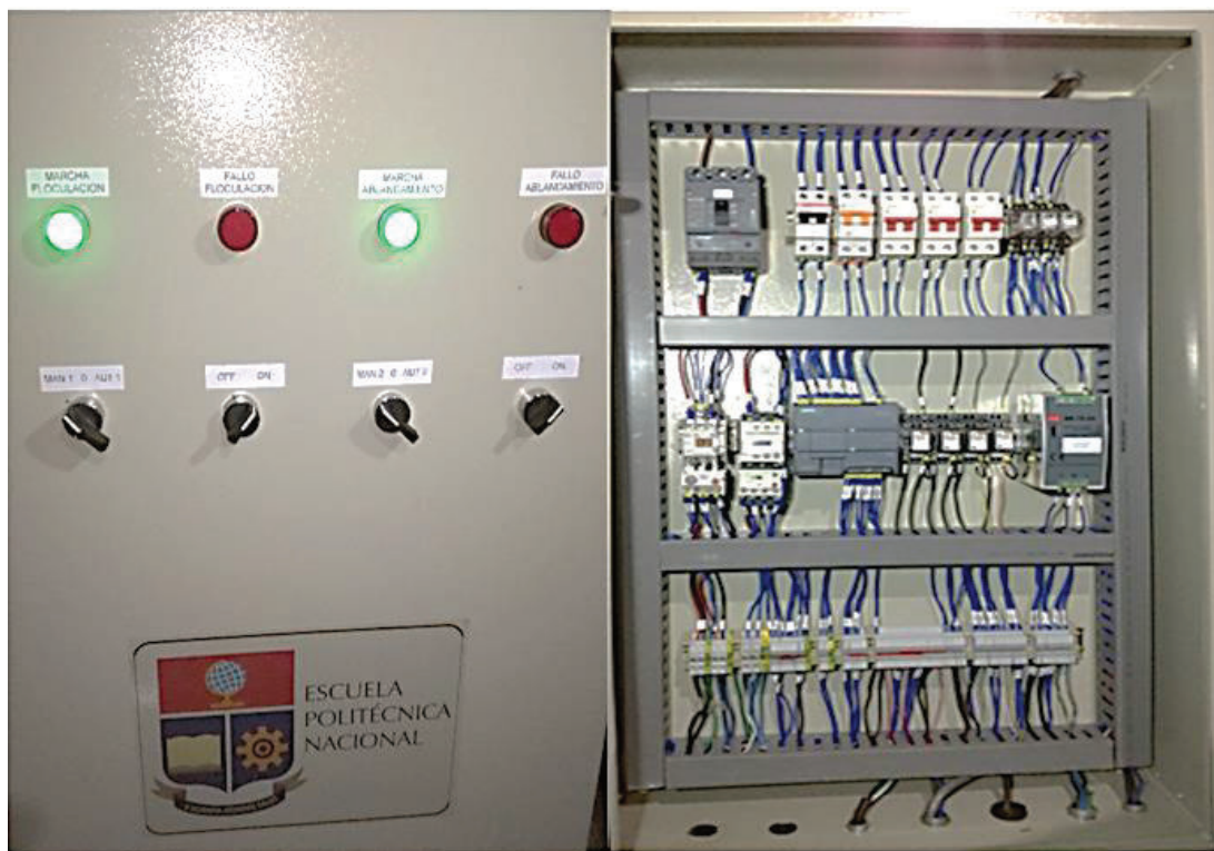
Figura 20. Tablero de Control Principal
