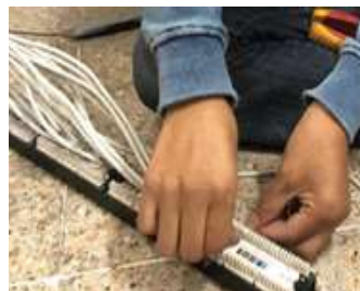
Figura 36 Ponchado Patch Panel
