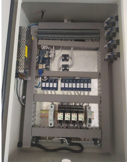
Figura 3.17: Tablero de control
