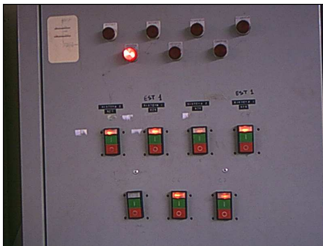
Figura 2.1 Tablero de control original
