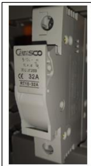
Figura 3.20: Base porta fusible.
