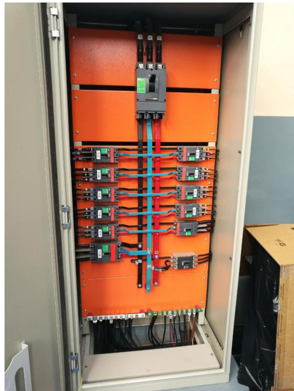
Figura 3.2: Tablero principal TP-T1
