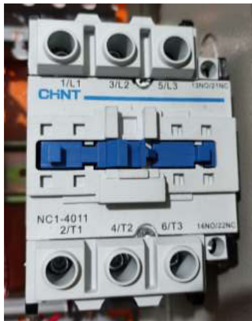
Figura 3.4 Contactor principal 40 (A).
