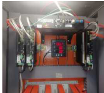
(e) Switches/Routers Garret-com
