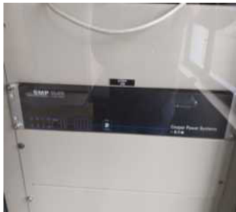
(a) RTU Cooper
