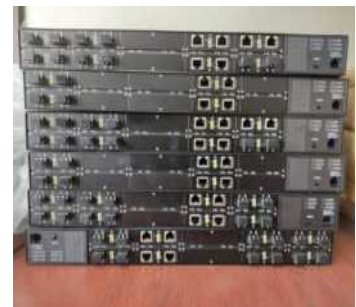
(f) Routers Ruggedcom
