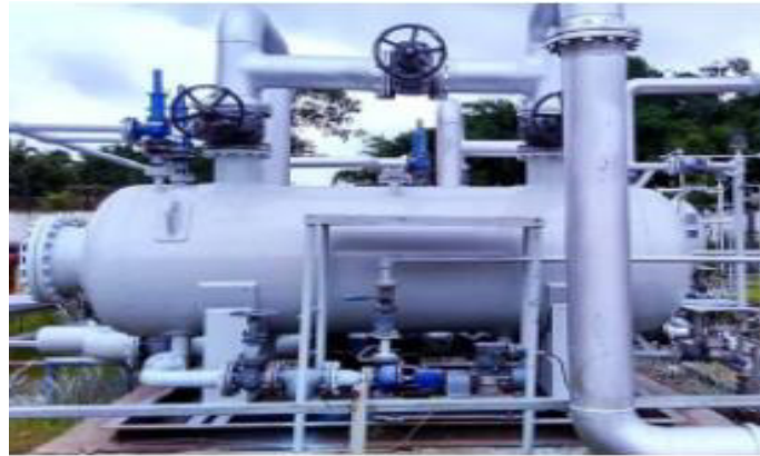
Figura 1.3. Knockout Drum horizontal (API 520, 2008)
