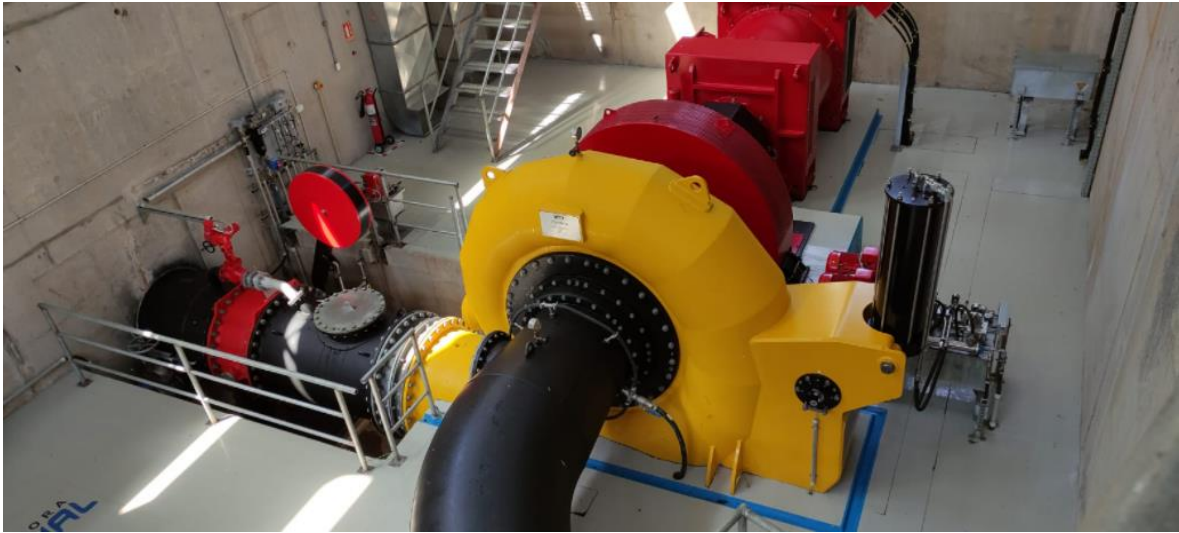
Figura 15. Turbina Francis central Palmira Nanegal.
