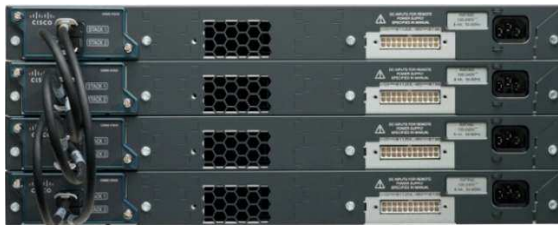
Figure 3. Cisco FlexStack Module and Switches
