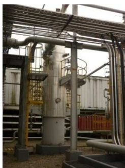
Figura 3.205: Scrubber de Gas Combustible
