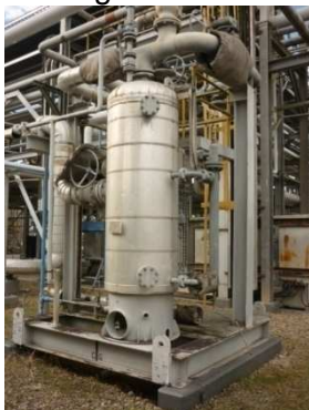
Figura 3.236: Scrubber de gas blanketing
