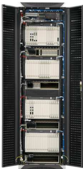
Figura 2.6 Softswitch Huawei SOFTX3000 [10]
