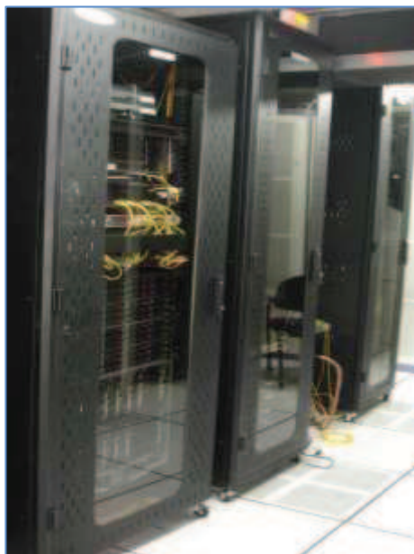
Figura 2.9 Racks de Gosseal
