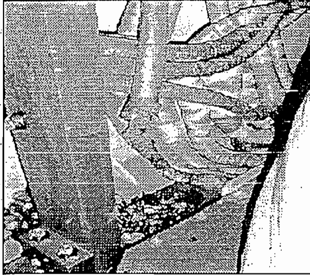
Figure 5 - Burnt HV Lead and Connector
