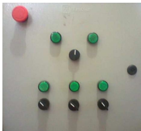
Figura 4.5 Panel de control
