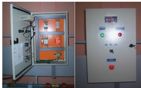
Figura 3.17 Tablero de control
