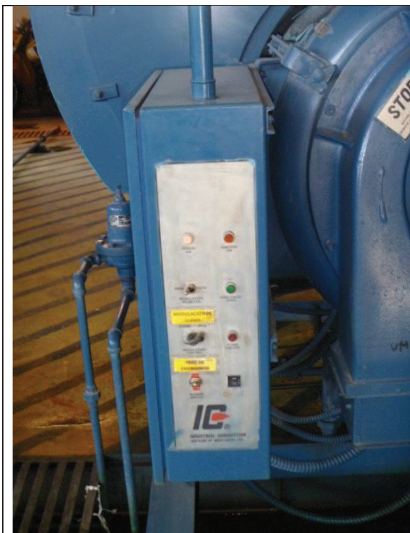
Panel de Control
