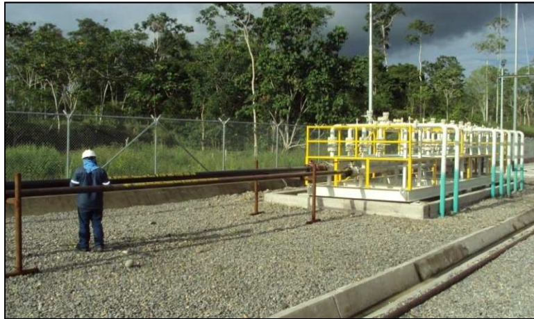
Figura 3.2 Manifold del Well Pad Sac-65B
