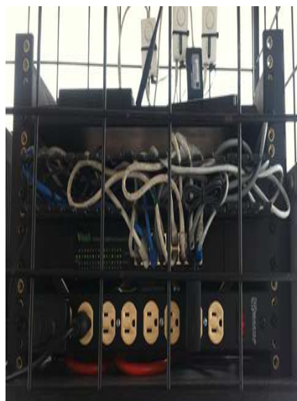
Fig. 3. 15 Rack Hospital Metropolitano
