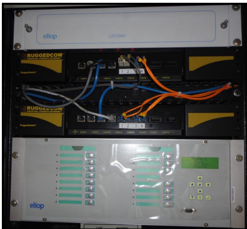
Figura 2. 34.- Vista Frontal Rack S/E Selva Alegre (Gateway, Switches y RTU)
