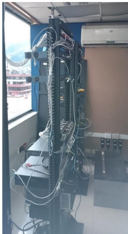
Figura 2.8: Racks LEVITON de ECUAONLINE S.A.
